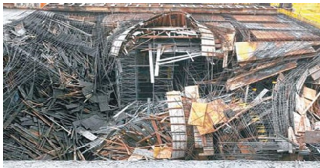
Figure 2 – Collapse of Falsework at Hong Kong Science and Technology Park Phase 3
