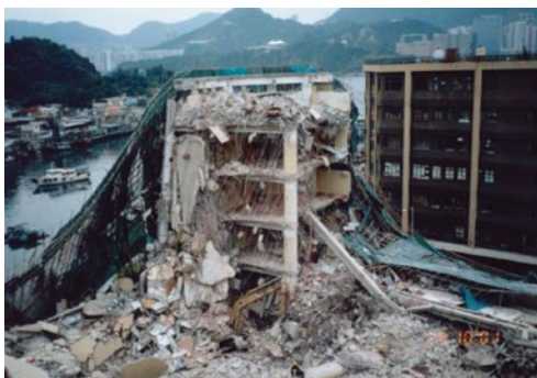
Figure 1 – Collapse of Falsework at Sze Shan Street, Yau Tong
