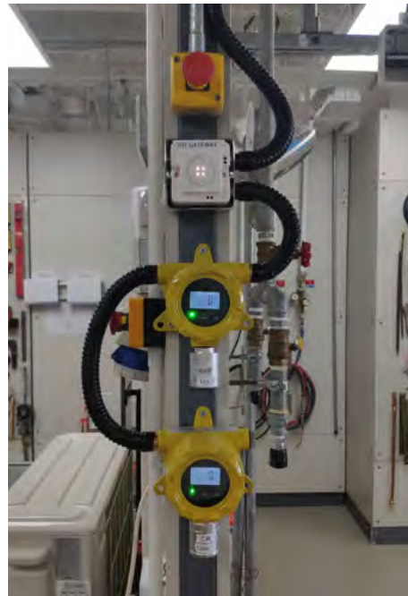
Additional IoT sensors at Hong Kong Construction Industry Trade Testing Centre (HKCITTC)
