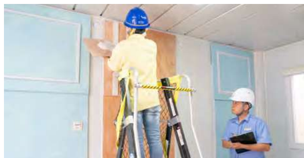
The San Tin Training Ground provides Intermediate Trade Tests for Painter and Decorator
