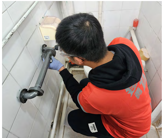
Construction Industry Volunteer Service Day - Construction Industry Volunteer Team installing handrails for elderlies
