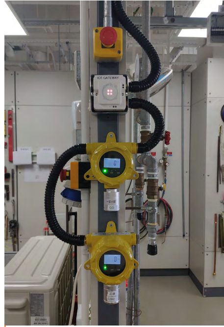
Additional IoT sensors at Hong Kong Construction Industry Trade Testing Centre (HKCITC)
