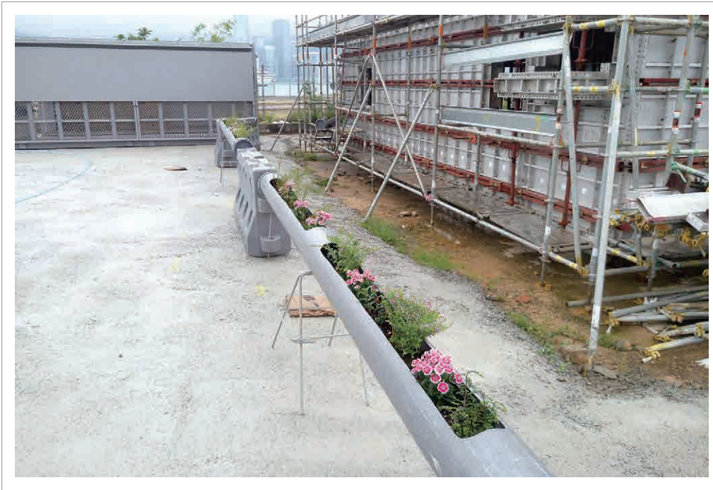
Old pipes and barriers are re-used for an integrated greening and barrier system in Wai Lok Street training ground 位於偉樂街訓練場的綜合綠化屏障系統，由循環再用的舊喉管和防撞欄組成
