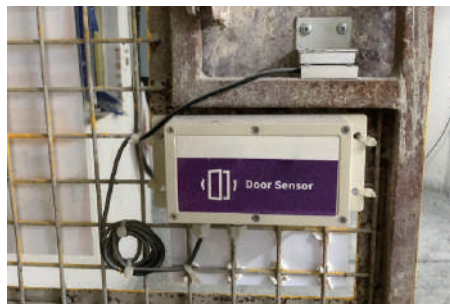
Hazardous Areas Access Control by Electronic Lock and Key System
