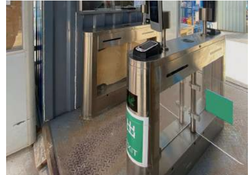
Install gate(s) with card reading device(s)
