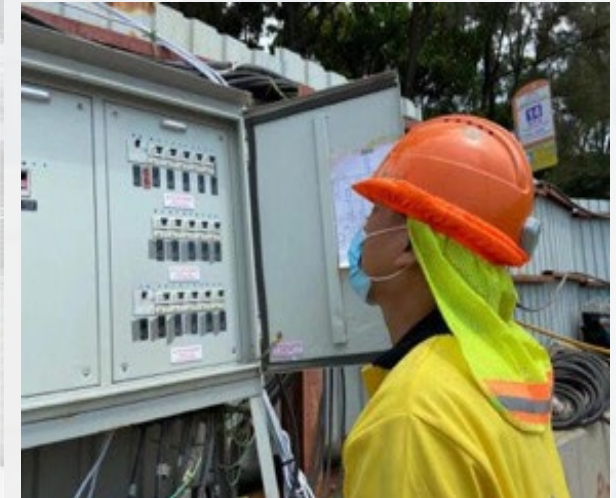
Electrical box opening management
