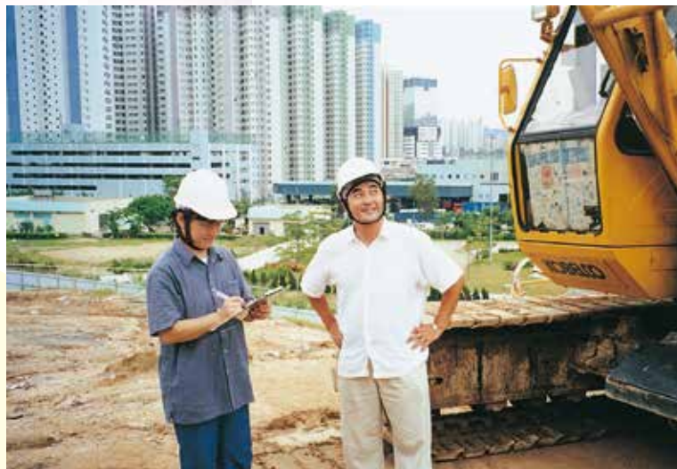
The site agent, through inspection programme, evaluates the effect of implementing 5S on a regular basis to decide on future improvements actions
