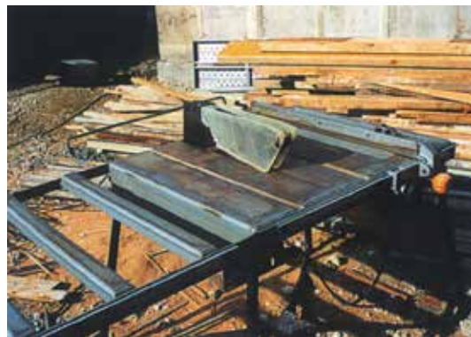
Transparent machine guards are used on machinery, making it convenient to check whether the equipment complies with necessary standards
